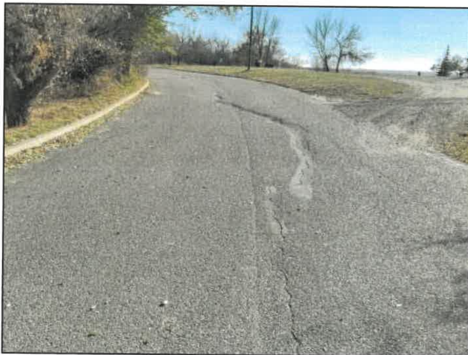
PHOTOGRAPH NO. 18533-06: Tension crack in roadway along east slope. Location approximately 300 m south of rail bridge.
