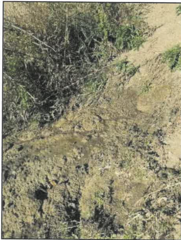
PHOTOGRAPH NO. 18533-10: Groundwater seepage face along slope, downslope of area shown in Photo No. 18533-09
