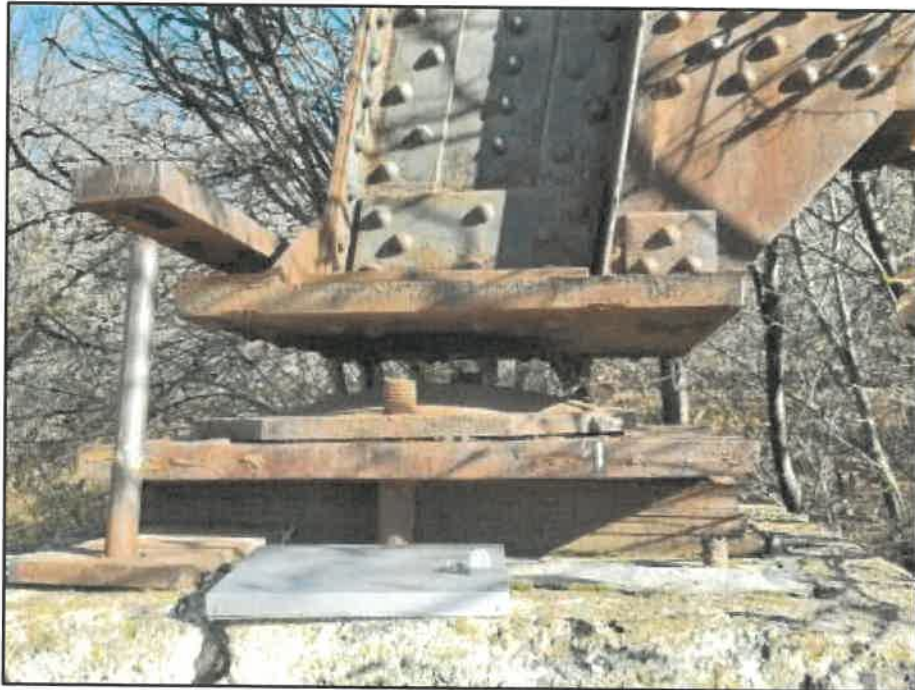
PHOTOGRAPH NO. 18533-02: Gap under bridge pier on east slope.
