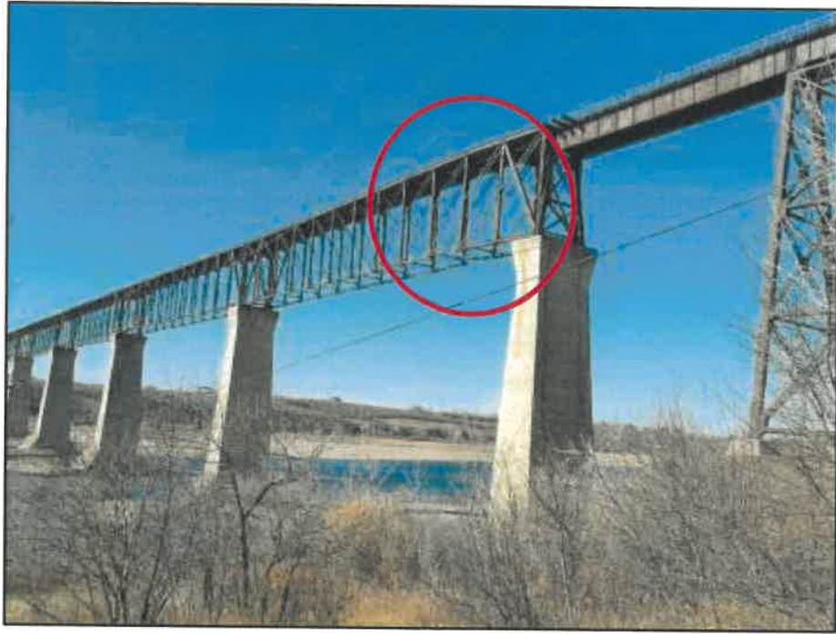
PHOTOGRAPH NO. 18533-01: Buckling of truss near the abandoned rail bridge pier along the east shore of the river.
