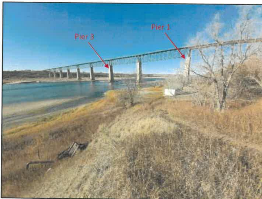
PHOTOGRAPH NO. 18533-04: Looking northwest towards proposed new raw water intake location (next to Pier 3). Pier 1 at toe of slope appears to have heaved upwards.
