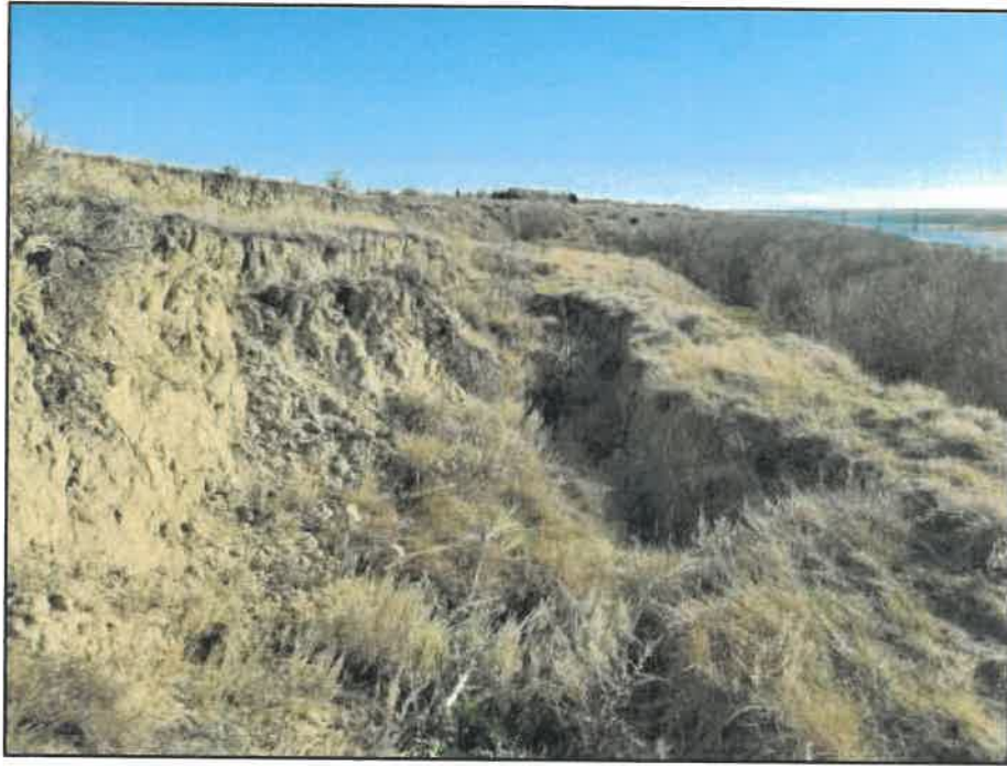
PHOTOGRAPH NO. 18533-09: Slumping and wide deep tension cracking along east slope, approximately 1.5 km north of rail bridge.
