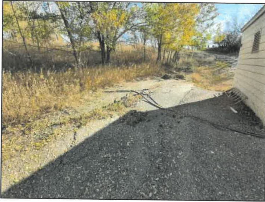
PHOTOGRAPH NO. 18533-07: Tension cracking around existing sewage pumpstation, located north of rail bridge east abutment.
